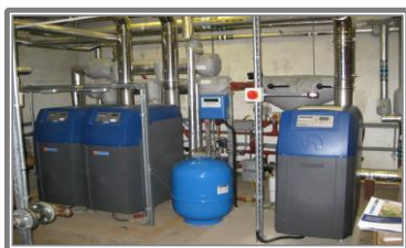
New high Efficiency Condensing Boiler – Norbury School
