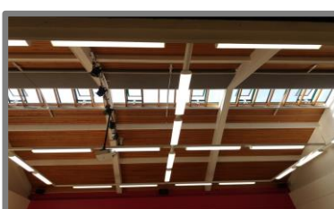
Whitchurch primary School – new LEDs
