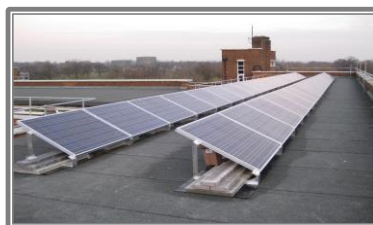
Renewable investment - Solar PV in Stanburn primary School
